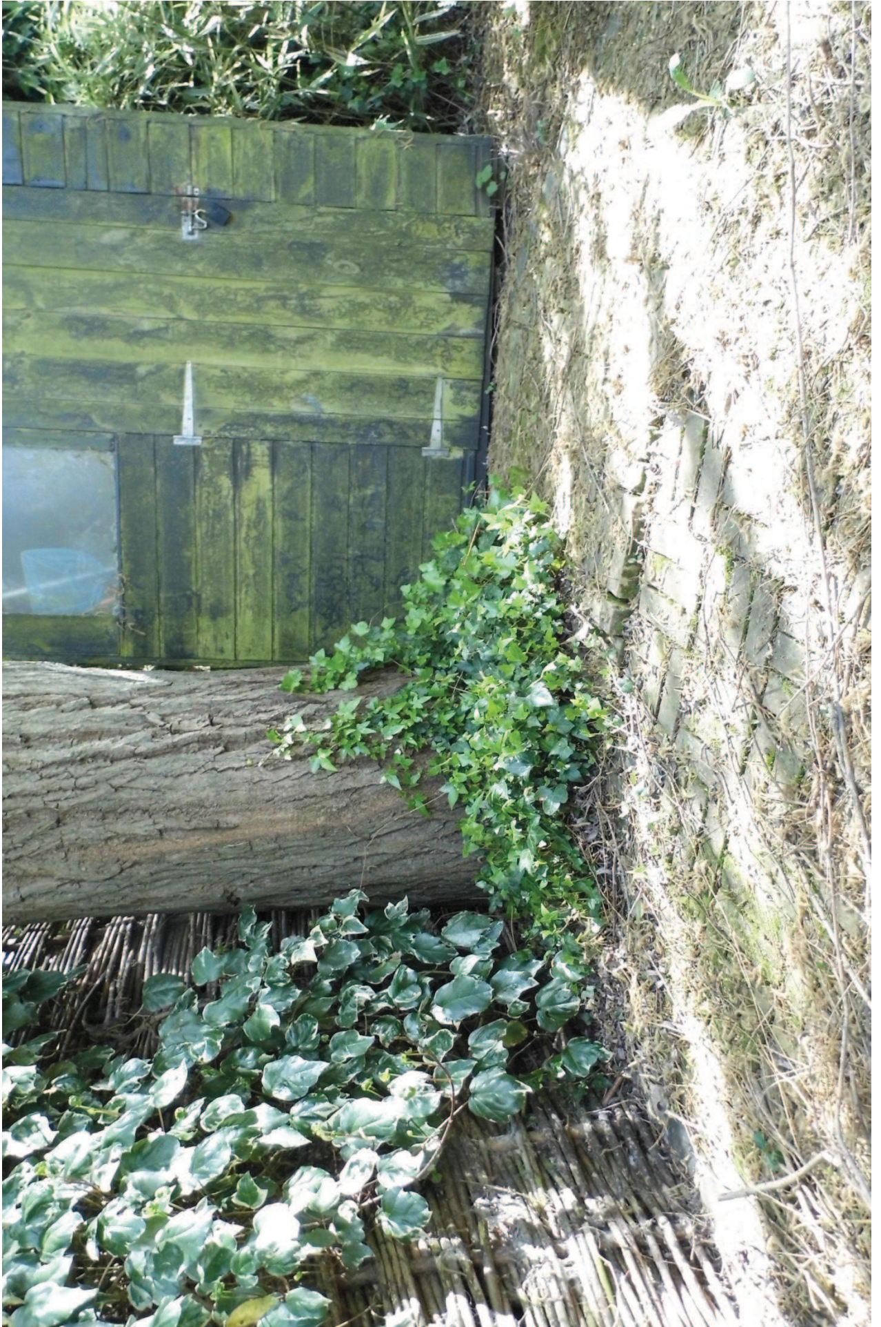
Paving and shed disturbed by tree roots
